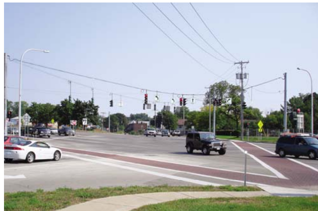
Installation of nonplanar slabs in intersection of Rt 7 and Watt Street, Schenectady, N.Y. (2006).
